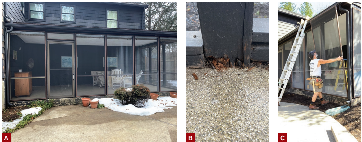
Figure 1. The roof of the existing screen porch was structurally sound (A), but the fir posts and sill plates were rotting where they were in direct contact with the porch's concrete slab floor and needed to be replaced (B). The aluminum screening in the aluminum-framed panels also needed replacement (C).
