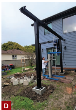
Figure 3. The homeowner (at center in photo) helps wrangle the first beam into place with the help of a Genie lift (A). The beam is bolted to the posts (B), then the second, longer beam is hoisted into place and secured (C, D).
