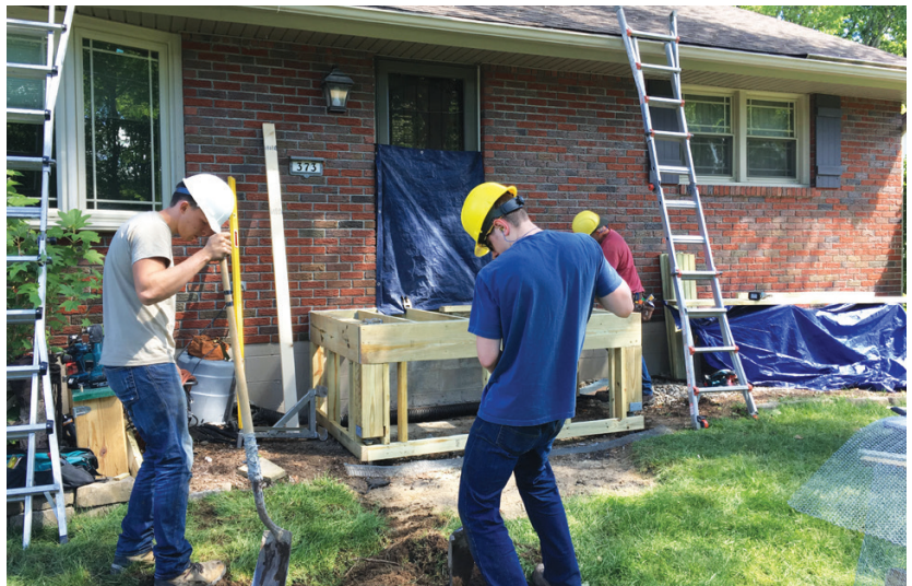
Figure 1. After the existing precast concrete stairway was removed, the author prepped the framing under the entry door to receive the new ledger (top). To keep rodents from burrowing under the enclosed porch, 12-inch-wide strips of diamond lath were nailed to the bottom of the framing and buried in the ground before the plywood sheathing was installed (bottom).
