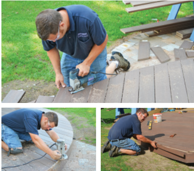
Figure 7. A worker laid out the curved portion of the decking, then carefully cut to the line with a jigsaw (top). Next, he smoothed the edge with a router equipped with a flush-cut bearing bit (above left), then covered the exposed end cuts with a second trim piece (above right).
