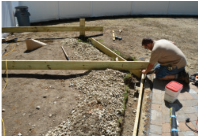
Figure 1. After digging a trench for the carrying beam, the crew used a hydraulic machine to drive helical piers into the soil until the required pier bearing strength was verified by the machine's on-board torque gauge (top). Adjustable-screw beam brackets set onto the steel-tube piers (above center) secure and support the built-up PT carrying beam (above).
