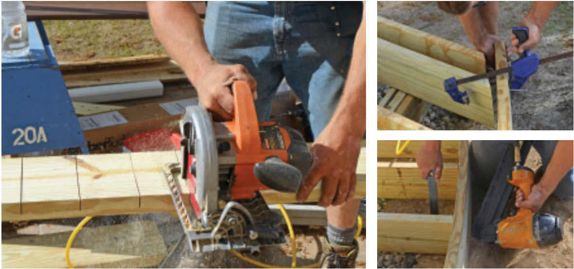
Figure 5. The band joist was framed with a pressure-treated 2x8 that was kerfed to allow it to bend and follow the curve of the deck (below left). With the joists resting loosely on the carrying beam, the crew clamped the band joist into position (below right) and nailed it to the joist ends before finally fastening the joists to the carrying beam (bottom right).
