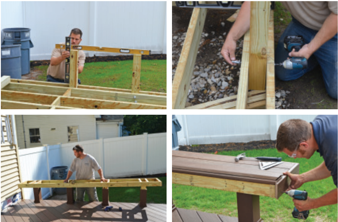
Figure 6. Along the high side of the deck, 4x4 posts support a bench, which serves a safety function in addition to providing seating (top left). After the posts were plumbed and fastened to the deck frame with ThruLok screws (top right), a ladder-framed bench structure was fastened to the post ends (above left). The bench was finished using the same Fiberon material used for decking and deck trim (above right).
