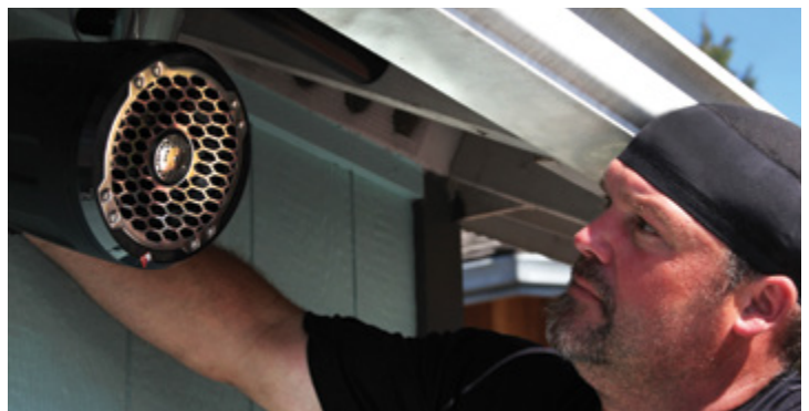
Figure 3. The author installed speakers designed for mounting on a wakeboard boat tower. The speakers are rated for full exposure to weather, with high-density polyethylene enclosures, and are equipped with adjustable aluminum hardware so they can be clamped to round rails.
