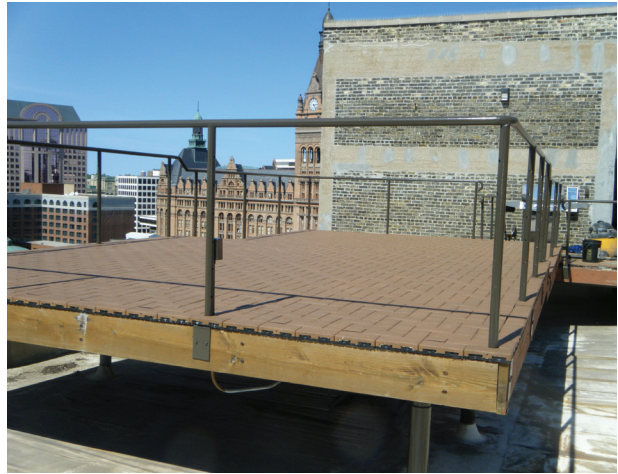
Figure 2. Faced with the logistics of transporting traditional decking in a freight elevator up to the roof of this downtown high-rise building, the author chose instead to resurface the deck with composite pavers.
