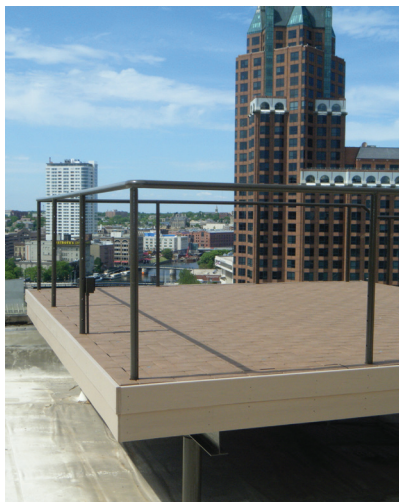
Figure 4. This deck was finished with a traditional two-tier fascia, which locks the pavers in place. The pavers were also glued to the installation grid to counter wind uplift.
