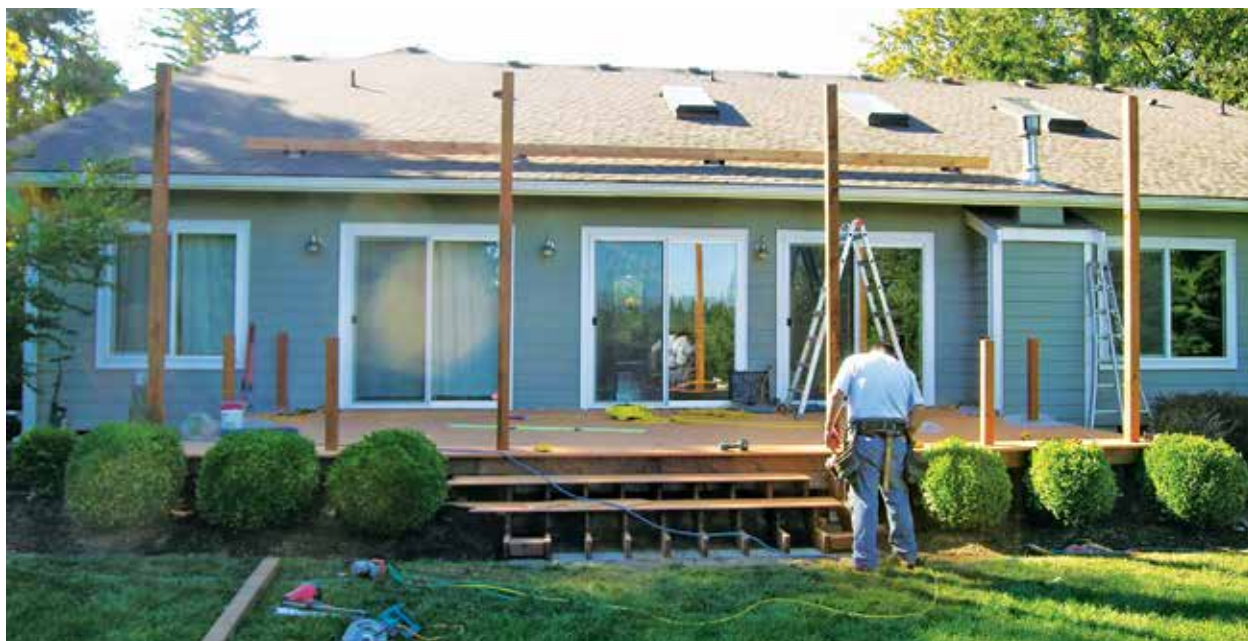
Figure 6. 4x4 posts bearing directly on the wall plate support the pergola beam located above the roof.
