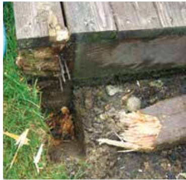
Figure 3. Fastening the treated rail posts directly to the framing created a collection zone where water and organic material were trapped, causing the adjacent wood to rot (top). The stair posts, which had been buried in the ground, had also rotted (above).
