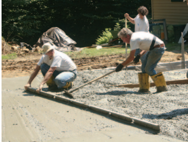
► Figure 11. Rakes, shovels, and “come-alongs” are used to move concrete into the forms and ahead of the screed.
