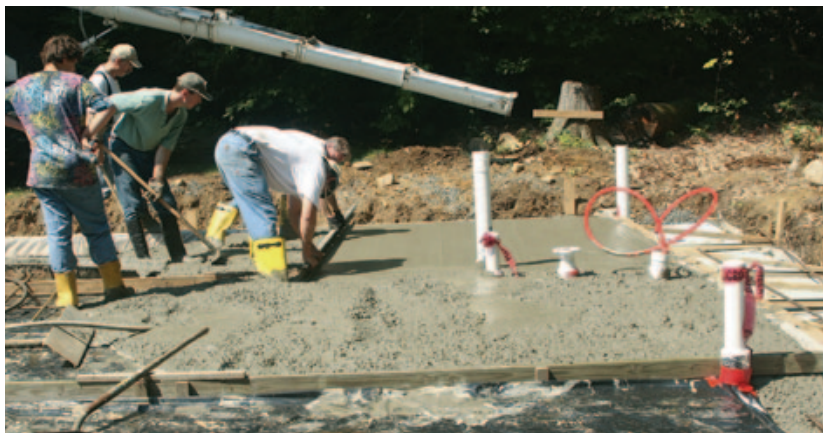
▼ Figure 10. For large slabs, intermediate screed supports are used. As the slab progresses, the screed supports are removed and the resulting voids are shoveled full of concrete.
