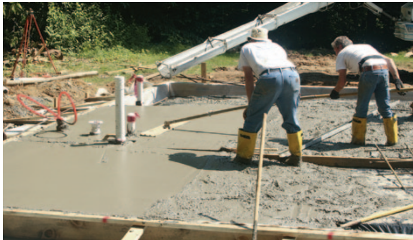
▲ Figure 12. After being screeded, large slabs are flattened with a bull float. Bull-floating also pushes the coarse aggregate down and brings up the finer, more easily finished “cream.”
