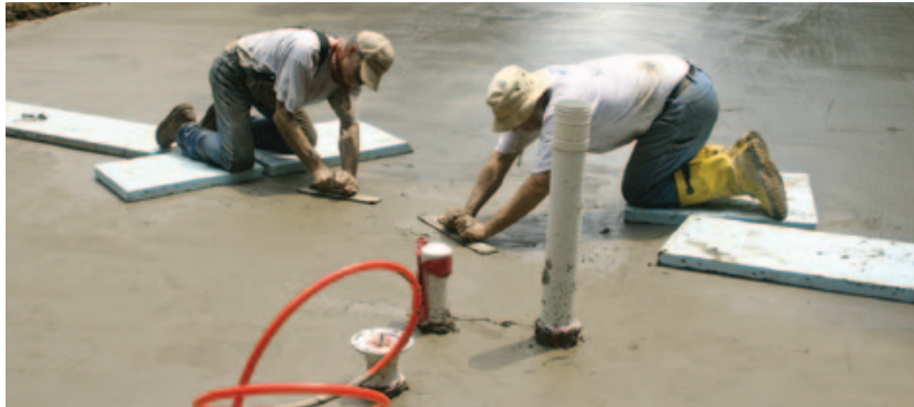
▲ Figure 18. Knee boards (here made of rigid foam, but usually of plywood) keep workers from sinking in the center of a large slab.
