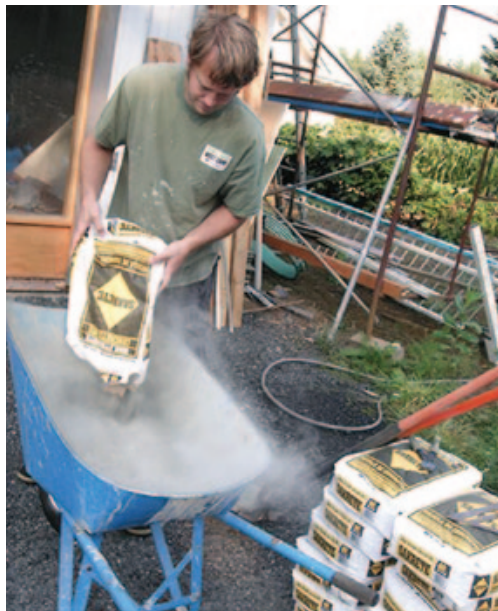
◀ Figure 1. The author finds that for less than one yard of concrete, site-mixing is cheaper than ordering it ready-mixed and paying short-load fees. Sixty 60-pound bags of concrete mix — enough to make a yard — at $2.90 each costs $174.
