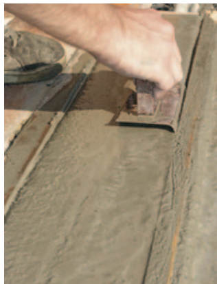
▲ Figure 14. Edging is a multi-step process that's repeated each time the slab is floated or troweled.
