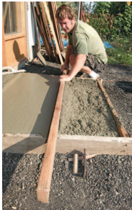
► Figure 9. Concrete is leveled by screeding — sliding a straightedge back and forth across the forms while moving it forward.
