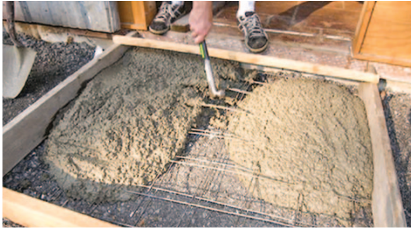
▲ Figure 8. Steel mesh needs to be pulled up when the concrete is placed so it ends up in the center of the slab.
