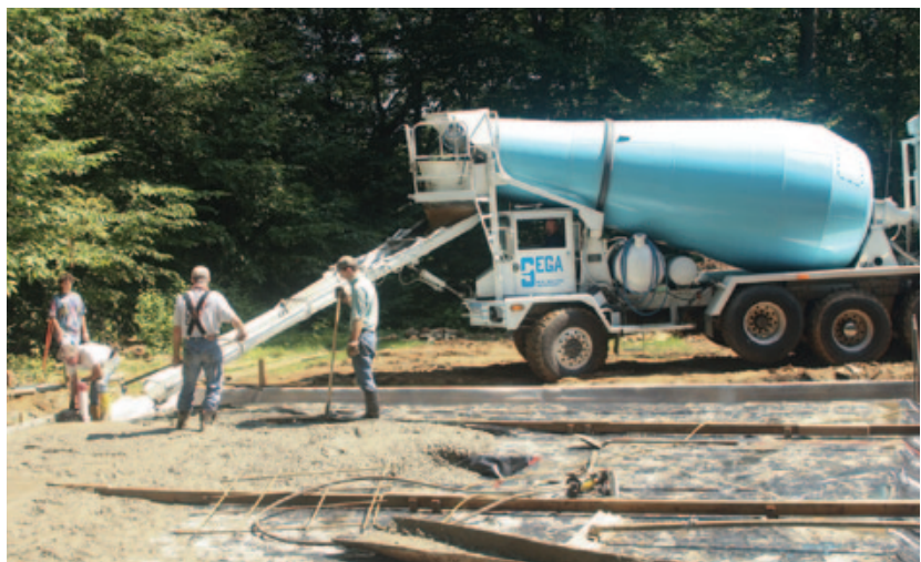
▲ Figure 2. Ready-mixed concrete at $85 per yard plus a short-load charge of $120 will run at least $205. It's not cost-effective for pours smaller than one yard, but it makes sense for larger pours.
