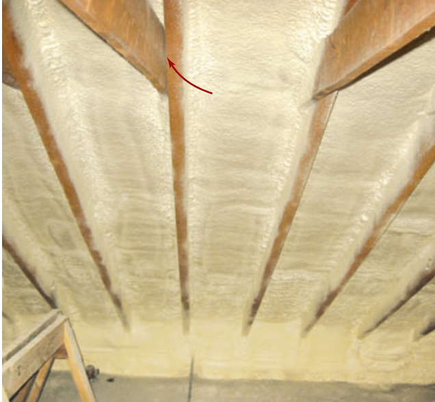
Figure 1. This correctly applied closed-cell foam has been sprayed directly against the underside of the roof deck. To eliminate air leaks at the eaves, the foam has been extended beyond the top plate to form a seal against the attic floor. One minor omission: An additional shot of foam to each of the cracks between rafters and collar ties (arrow) would have prevented any possible air movement through that interface.
