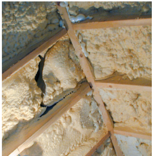
Figure 3. Closed-cell foam applied in lifts that are too thick is subject to overheating, which can lead to subsequent shrinkage and cracking — a problem that may not become evident until months after the applicator has packed up and left. The lighter-colored areas of foam mark the location of cracks that had been filled in an earlier attempt at repairing the still-ongoing shrinkage (top). Cracks in the foam sprayed against the roof sheathing precisely matched melted areas of frost on the roof exterior in cold weather. Because such cracks may extend all the way to the sheathing, humid indoor air that moves through them may condense on the cold underside of the sheathing, promoting mold growth or rot (above).
