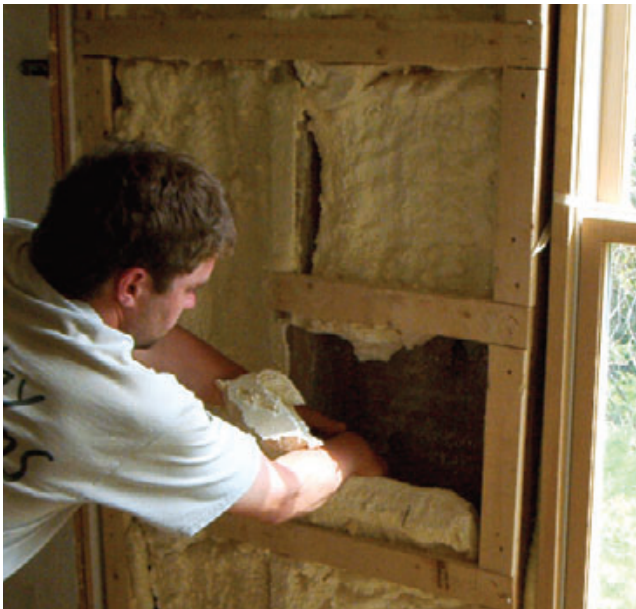
Figure 2. Defective B-rich foam, like that shown here, is characteristically soft and sticky and has a distinctive chemical odor. The material has not bonded to the sheathing beneath and can easily be pulled from the framing cavities by hand.
