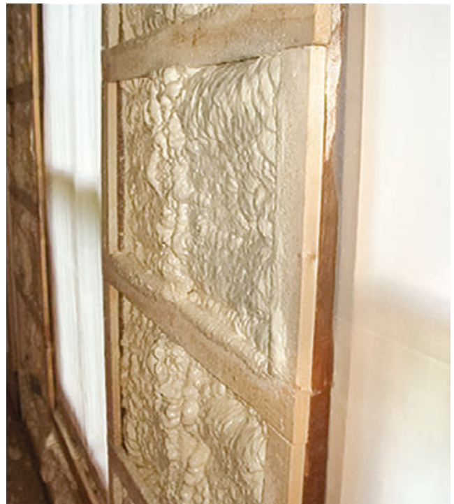
Figure 8. Depending on the R-value required, open-cell foam can be applied to a depth greater than the framing before being trimmed back flush (top). Denser closed-cell foam is much more difficult to trim. By allowing the foam to extend beyond the plane of the framing (above), this installer has created a major headache for the drywall crew. The author's tool of choice for trimming limited areas of closed-cell foam is an angle grinder fitted with a coarse 6-inch steel cup brush.
