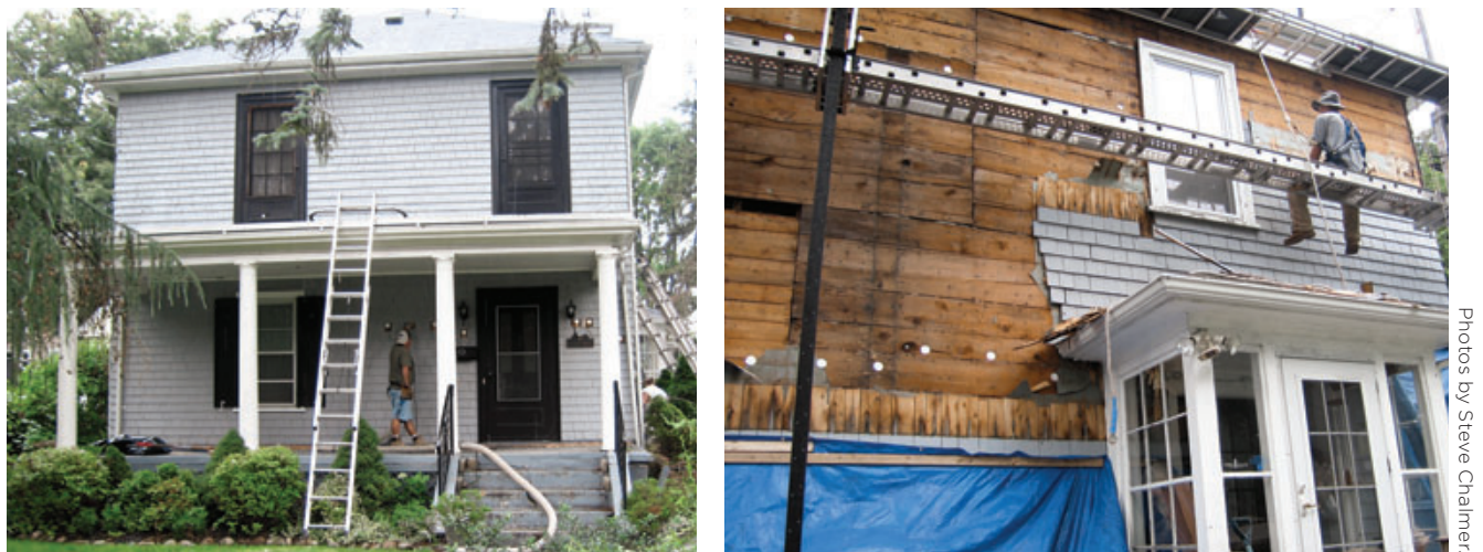
Figure 2. The wall cavities were first dense-packed from the outside with blown cellulose insulation (left). Then the crew stripped off the old cedar shingle siding, focusing on one side of the house at a time to protect the exposed walls and insulation from the weather (right).
