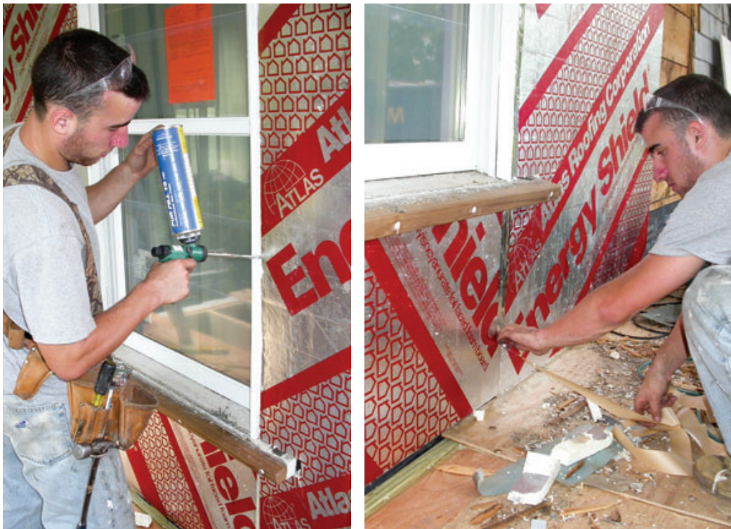
Figure 4. The walls were wrapped with 1-inch-thick sheets of polyisocyanurate foam, which adds R-6 to the wall assembly and acts as an air and vapor barrier and drainage plane. All joints — including gaps between the rigid foam and jamb extensions — were foamed (far left) and sealed with flashing tape (left).
