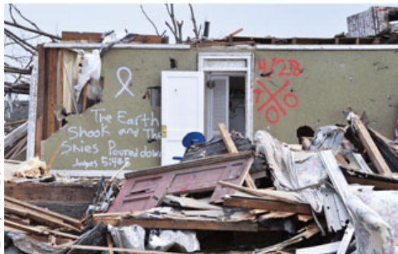
The wreckage of this home, in the aftermath of a tornado that struck Tuscaloosa, Ala., on April 27, demonstrates the tendency of some interior rooms to remain largely intact even when the rest of a structure has been demolished.
