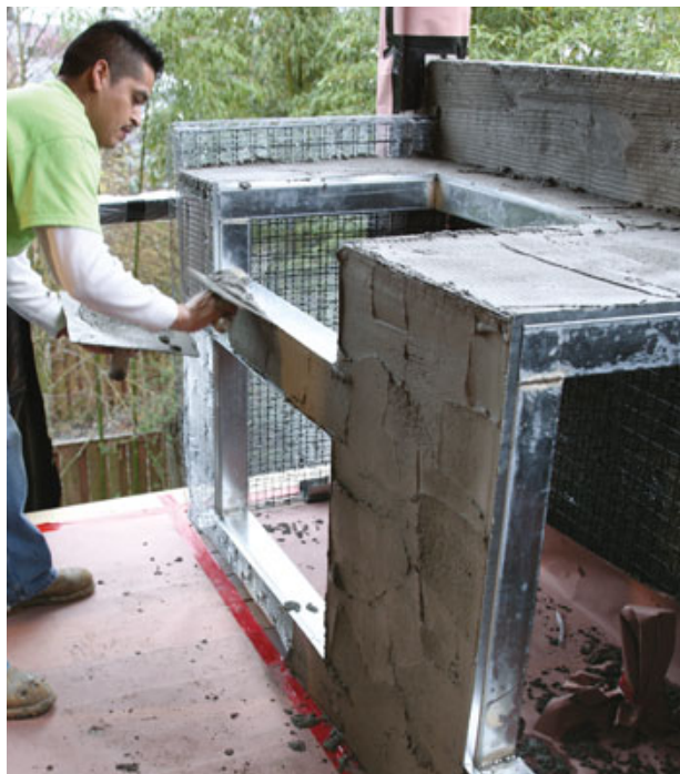
Figure 6. Once the panels are covered with wire lath, a traditional stucco or man-made stone finish can be applied.
