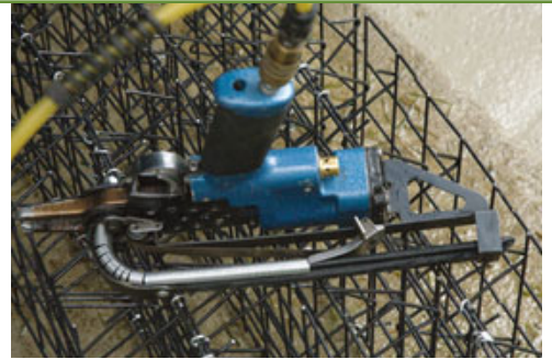
Figure 4. A special tool rented from Galvacore joins together panels with wire rings.
