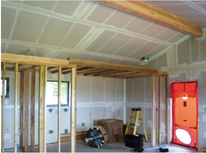
Figure 9. A drop ceiling above interior partition walls (left) provided space for the ERV and associated duct-work (below left). A furred-out wall on the north side of the kitchen and utility room — completely within the air-sealed thermal envelope — made it possible to run pipes and wiring as needed without additional air-sealing or insulation (below).
