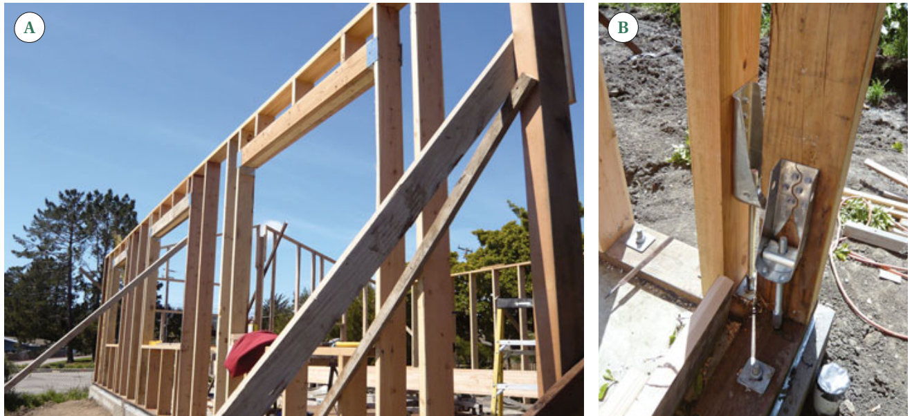
Figure 3. Insulated headers supported by metal connectors are a hallmark of OVE framing (A). Though framed with less lumber, the shell meets West Coast seismic requirements (B). To eliminate air leakage at the ridge, the crew installed blocking between the rafters, sealing it to the framing with spray foam (C). The blocks (D) were ripped so they could be caulked into place, bearing solidly on the glulam beam and matching the angle of the rafters to provide a caulkable nailing surface for the sloped ceiling drywall.
