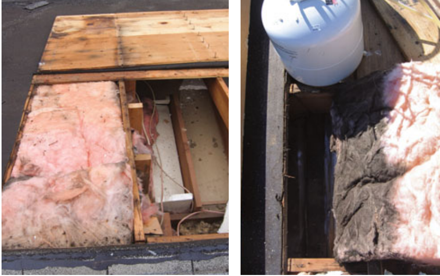
Figure 4. At the interface between the addition and the original attic, warm, moist air flowing through the batts in the cathedral ceiling had been condensing on the sheathing, rusting the nails and staining the plywood (left). Along the addition's ridge, air leaking from inside had left a dirty deposit in the batt insulation (right).
