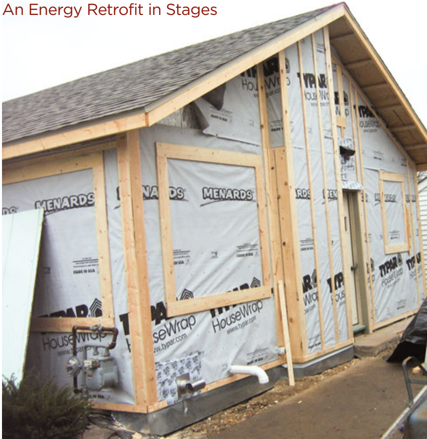
Figure 8. After dismantling the old gable-end chimney above the roofline, the crew enclosed the lower part in a framed, insulated bump-out. The vertical strapping over the bump-out — not yet complete on the rest of the wall — is a rain-screen nailing base for horizontal fiber-cement siding.
