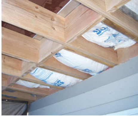
Figure 3. Running the deck joists inside the cantilever to bear on the mudsill is viable. Solid blocking has replaced the original band joist, and the insulation has been replaced. Remaining to be done is replacing the covering below the cantilever and waterproofing the joint between the deck joists and the exterior cladding.
