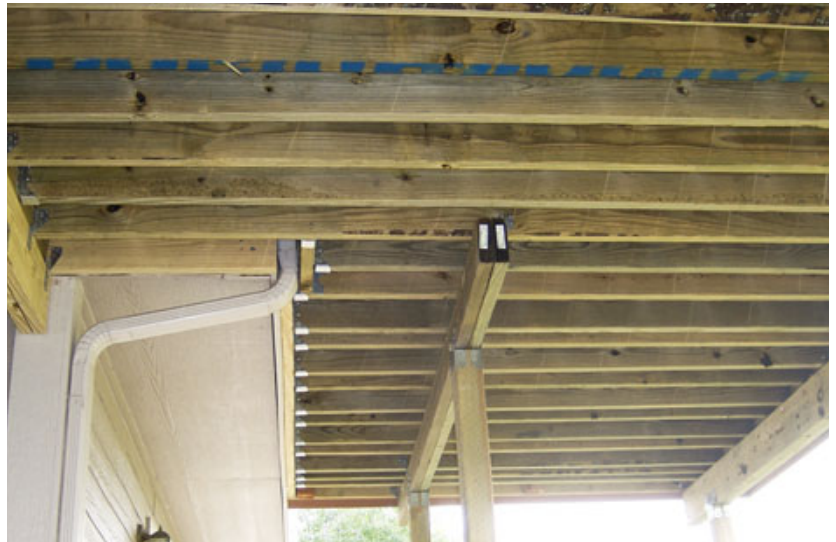
Figure 1. One approach to framing decks around a cantilevered floor is to add posts and a beam, then cantilever the deck itself back toward the cantilevered portion of the house.
