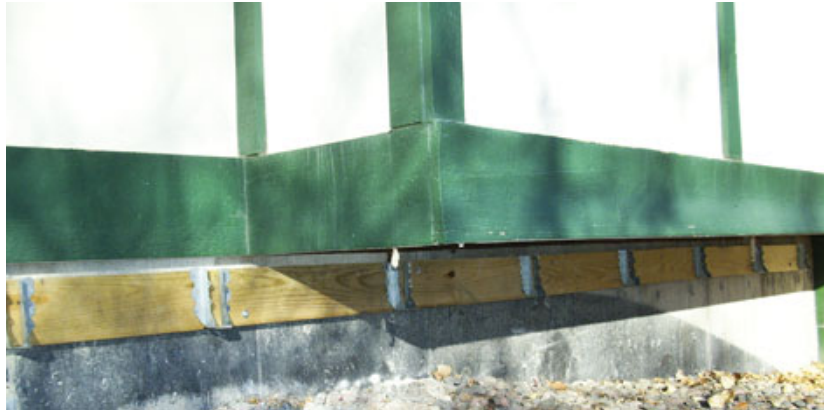
Figure 2. Sometimes you can bypass a cantilever by placing the ledger below it.
