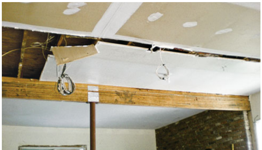
Figure 5. Before removing the improperly supported bearing wall in the family room, the GC built this temporary support wall (top). Note the wide bottom plate, meant to spread the load as much as possible over the settling slab. Once the bearing wall was gone, a pair of glulam beams was installed overhead, supported at midspan by a steel post on a new footing (above).
