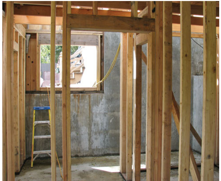
Figure 8. With the new foundation in place, framing continues (top left). The proximity of mature trees testifies to the care the author took to blend the building sensitively with the site (top right). The retaining wall foundation adds needed living space where the building steps down the hillside (above).
