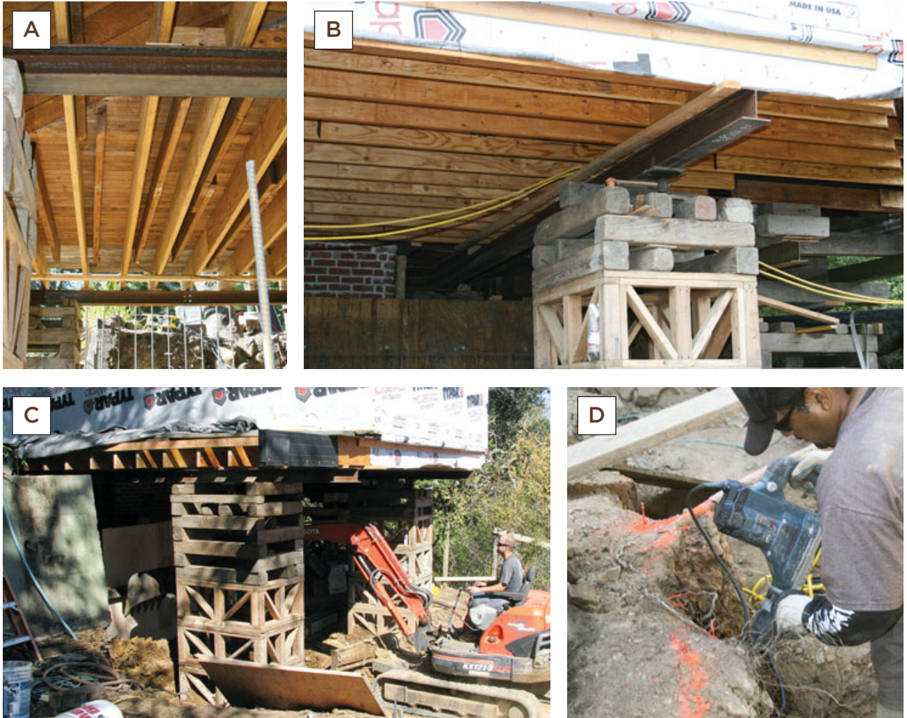
Figure 2. The author’s crew reinforced the existing underframed floor system with full-span LVLs (A, B). This allowed the cribbing and shoring contractor to support the entire house frame with several long steel I-beams, so that excavation under the house could proceed — a combination of mini-excavator work (C) and hand-digging. Here (D), a worker uses a rotary hammer with a spade bit (E) to cut through the hard, gravelly soil.
