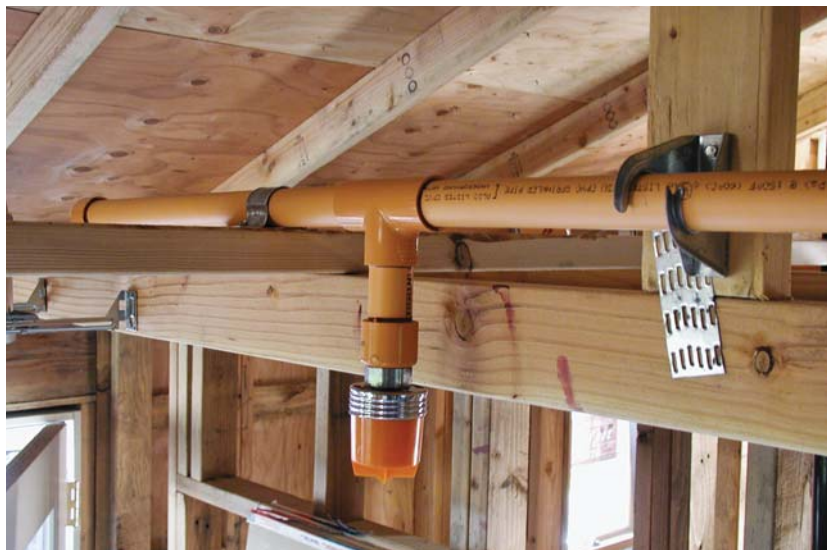
Figure 5. CPVC pipe flexes enough to be pulled into joist bays (top), where it can be glued and then inserted into fittings (center). The system above has been tested for leaks and is ready for drywall to be installed. The head is covered by a protective plastic cap, which will be removed after painting and replaced with a trim piece or cover plate.
