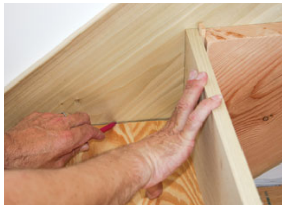
Figure 3. Tracing a mockup of an assembled tread and riser onto temporarily installed skirtboards lets the author transfer the rough stringer profile to the finished layout, ensuring a precise fit.
