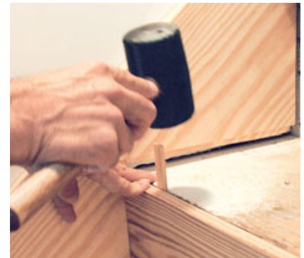
Figure 7. A fully sheathed rough carriage requires a different approach. The skirtboards are cut to fit the stair profile. On this stair, the author opted to house the treads only and scribe-fit the risers between the skirt faces. Shims force the riser to lock onto the tread. Treads must be shimmed from the front to snug them up in the housings.
