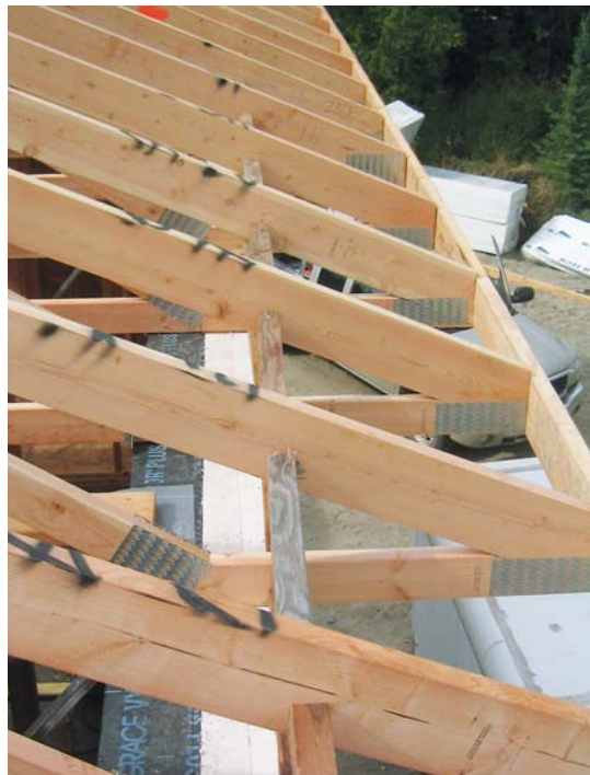
Figure 5. To ensure the continuity of the barrier membrane and exterior insulation, the wall to the right of this garage roof was covered with poly and foam before the roof was framed (top). Moving truss blocks in line with the outer edge of the exterior EPS will allow the cellulose in the attic to completely cover the full thickness of the exterior walls (above).
