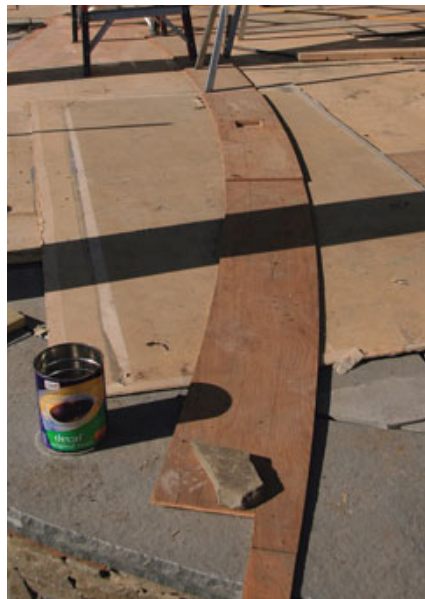
Figure 3. Identical plywood layout templates ensured a perfect match between site and shop efforts. The square cutouts pinpoint column centers.
