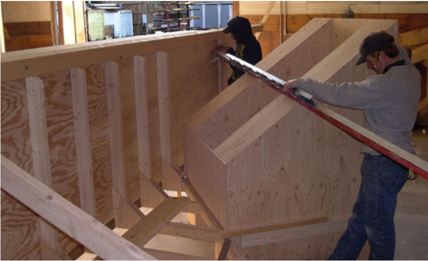
Figure 6. A plywood mockup of the existing roofline furnishes the correct cut angle for the roof intersection.
