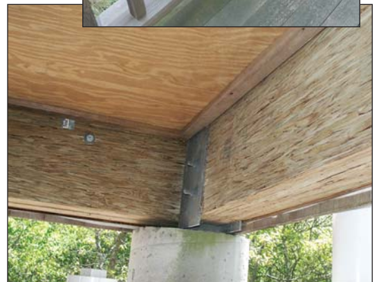
After 15 years in service, treated Parallam posts supporting a three-story beach house deck are as good as new (top). Treated Parallam girders supporting the main house's first-floor system likewise show no ill effects from weather or insects (bottom).
