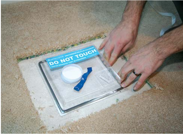
Figure 1. The author uses the calcium chloride test to check the slab for moisture. Dry calcium chloride is weighed, sealed under a dome for a specified time, then removed and reweighed. The weight gain is used to calculate the moisture vapor emission rate (MVER) of the concrete.
