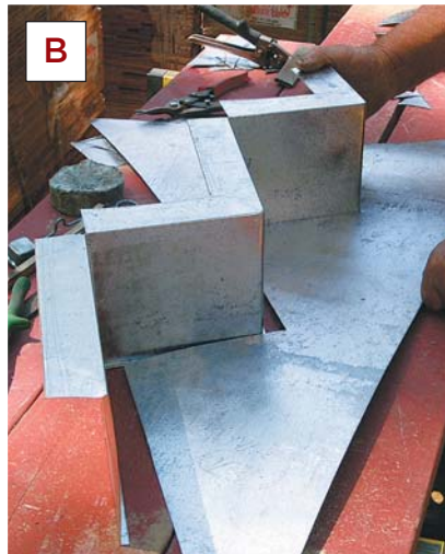
Figure 3. Fred fabricates the through-chimney counterflashings on a bench at the site, cutting and bending and then fitting (B) and soldering (C) the side pieces.
