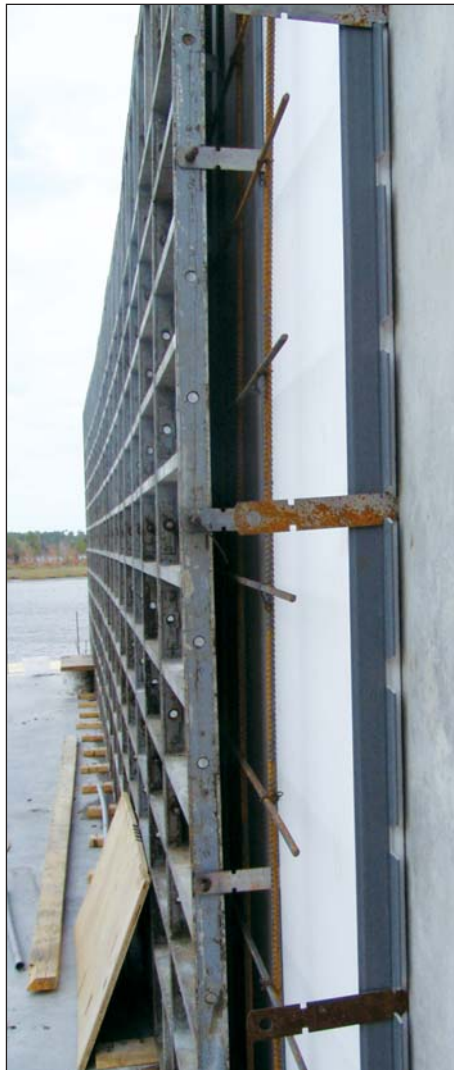
FIGURE 4. Workers start to form walls (far left) for a "housing lift" pour. Note the exterior wall forms, foam insulation, form spreaders, rebar, and door blockout. The spreaders lock inside and outside wall forms (left) together and hold foam tight against the outside face. Plastic nailer strips are locked into a slot routed into the foam.
