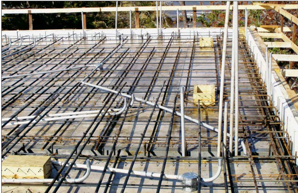
FIGURE 6. Prepping the slab formwork is laborious and exacting. Wiring conduit has to be carefully positioned within the dense mat of heavy rebar (left). The treated-wood blockout for an air-duct register has screws in the back to lock it to the slab, and is chamfered at the bottom so that the exposed-wood edge will be narrow enough for the grille flange to cover. Plywood caps on the wood blockouts raise them to a good height for use in guiding the screeds used to strike off the fresh concrete slab.
