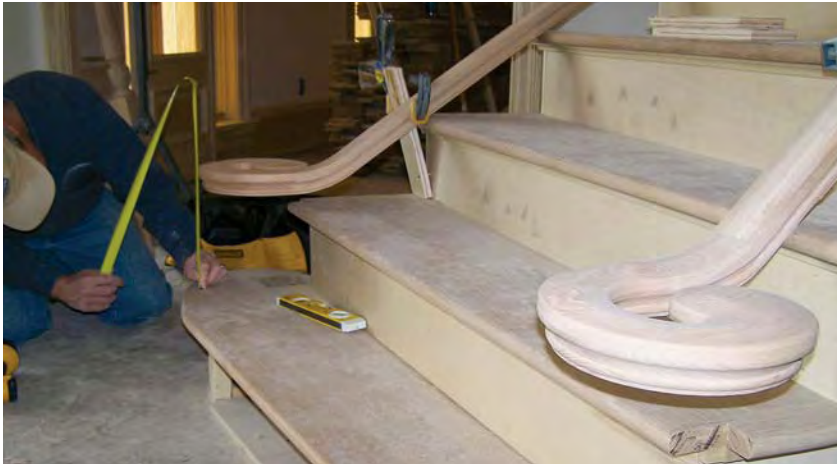
Figure 7. Measuring and fitting components is easier with the rail clamped firmly in place on the treads (left); after the newels have been installed and the rail lifted into position, a laser is handy for transferring the baluster layout to the underside of the handrail (below).
