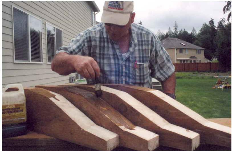
Figure 5. Cutting timbers usually exposes an untreated core. For longevity, coating all cuts in pressure-treated wood with an end-cut preservative is crucial.
