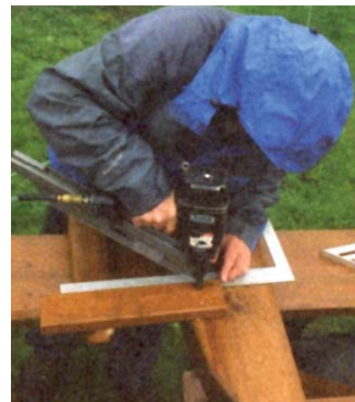
Figure 7. The author uses a framing square to be sure the seat-support 2x4s are at the correct 5-degree angle — which is a 1-in-12 pitch — as he nails them to the 4x10 posts.
