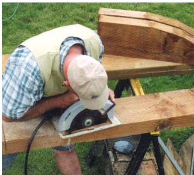
Figure 2. The back posts are laid out next to each other on 4x10 stock, minimizing waste. Cutting such thick material requires a 10-inch circular saw; the author will finish the cuts using a reciprocating saw.
