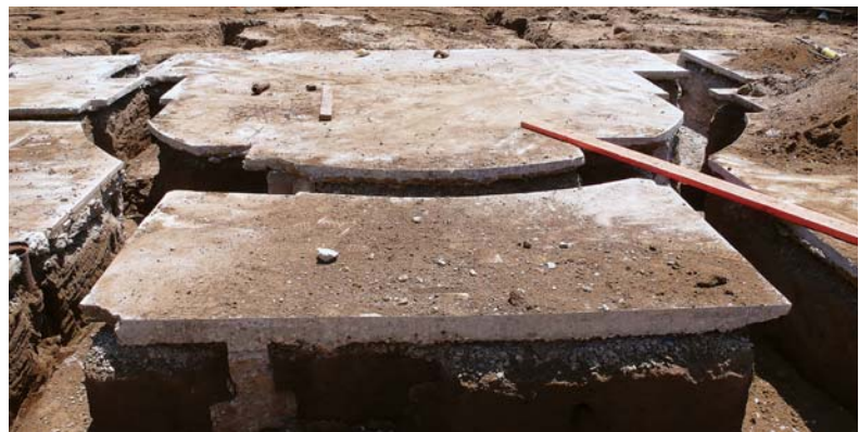
Figure 2. Extensive saw cuts indicate the positions of new footings within the original slab (top); the trenches continue into the surrounding soil. The semicircular cut (above) is intended for a stem wall to support two curved stair risers.
