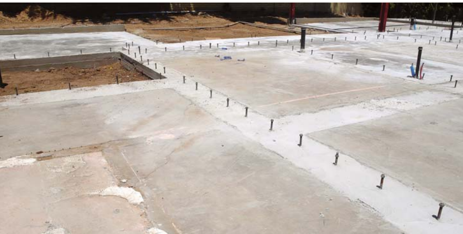
Figure 7. Once all the rebar and subslab mechanicals were in place (top), it took three days to pour the entire slab (above). After framing is complete, a lightweight concrete topping will eliminate surface irregularities in preparation for finish flooring.
