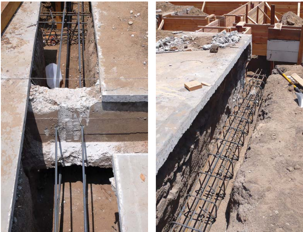
Figure 3. Where existing footings intersect the new trenches (far left), deeper footings underpin the old work, and continuous rebar passes right through the concrete to unify the structure. To carry exterior wall loads, perimeter grade beams require #5 rebar cages and a 3,000-psi concrete mix (left).
