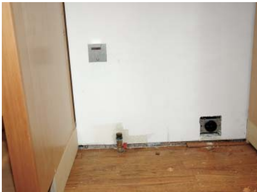
Figure 2. The rough-in for a dual-fuel range includes a 220-volt outlet, a gas connection with shutoff, and — farther up the wall — a clip to prevent tipping.
