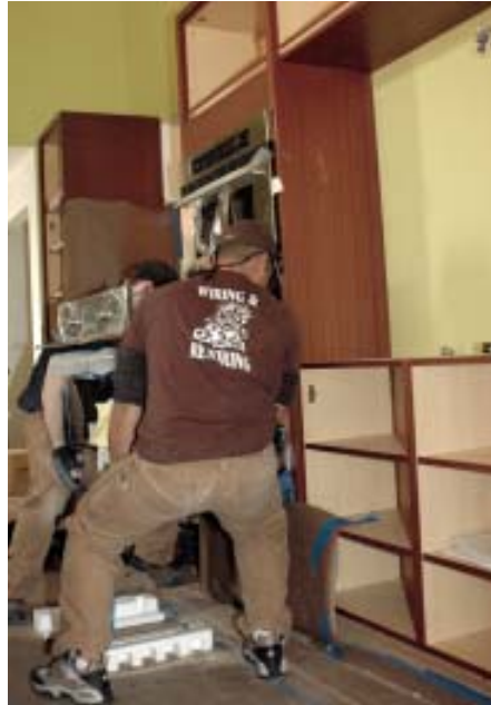
Figure 5. An electrician makes the 220-volt connection to a built-in convection-microwave oven (far left). The electrical box will be mounted in the back of the cabinet, which will also contain a conventional built-in oven, shown here (left) being lifted into place.
