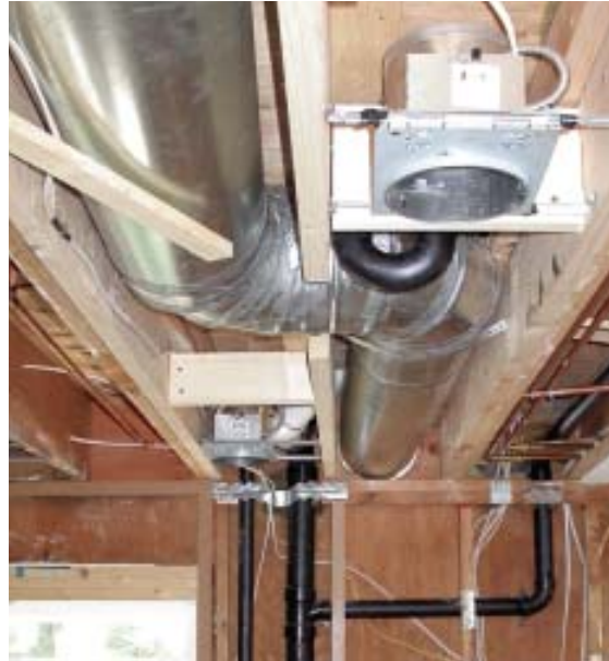
Figure 9. It's easiest to run an exhaust duct through unfinished attic space (far left). Ceiling runs are harder (left); to avoid lights and plumbing, this 10-inch duct had to jog between bays and through a joist — necessitating an engineered design that involved doubled \frac{3}{4} -inch sub-flooring above, and several sistered members.
