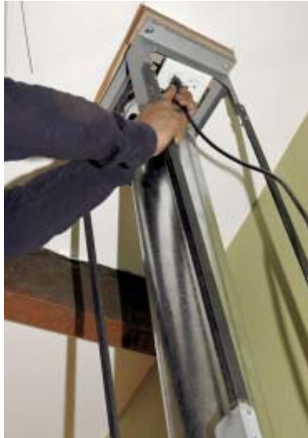
Figure 7. Since this vent hood wasn't tall enough to reach the ceiling, the author extended it with metal angles and a vertical run of duct (far left) that will be hidden behind a custom-fabricated cover. The hood plugs into an outlet in the ceiling above (left).
