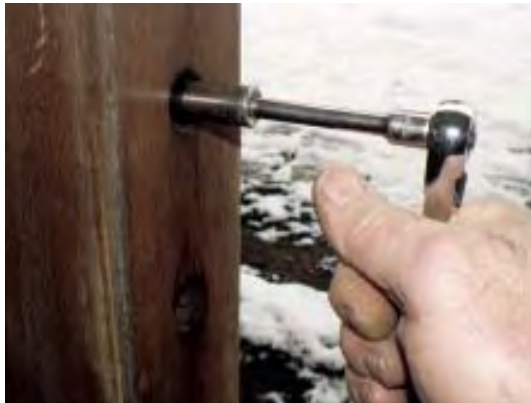
Figure 11. A two-step hole makes room for a socket wrench. The cable and stud enter the opposite side of the post through a smaller hole, and the nut used to tension the cable is buried inside a \frac{5}{8} -inch-diameter hole that also accommodates the socket.
