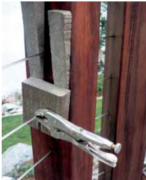
Figure 13. To pretension the cable before final tightening, the author uses locking pliers to grip the cable, and wedges to stretch it. He does this at several spots along a run, particularly at corners.
