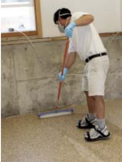
Figure 5. A clear top coat protects the chips and makes the garage floor shiny and easy to clean. It's mixed and applied in much the same way as previous coats, except it's poured directly on the floor and spread from there. Rolling the entire floor front to back and then side to side ensures uniform coverage with no lap marks.
