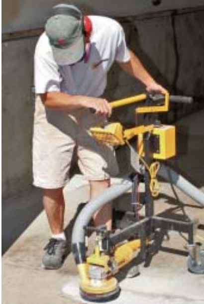
Figure 1. To prepare the garage slab for a two-part polyaspartic coating, the author grinds the surface with 50-grit diamond pads. He uses the larger machine (previous page) in the field and the smaller one (above) around the edges and on the sloping apron near the overhead door. Both are connected to a high-performance dust-collecting vac.
