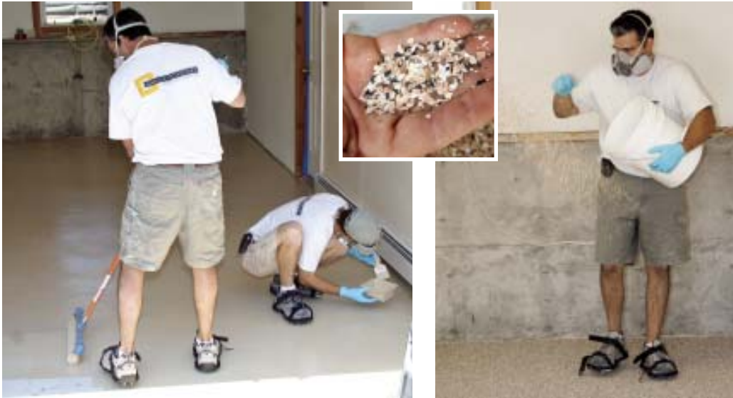
Figure 3. The two-part polyaspartic coating is applied with an 18-inch roller and cut in with a 3-inch chip brush (far left). Once the second coat is half done, the author starts spreading the vinyl chips (inset) that give the floor its distinctive look and dirt-hiding qualities (left).
