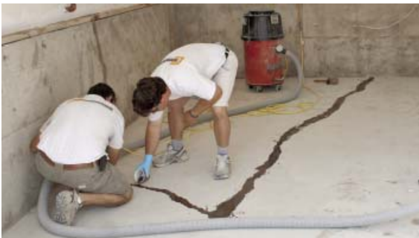
Figure 2. Workers fill cracks and pockmarks with silica sand, then pour on a rapid-setting two-part compound (above). After it dries — which takes only a few minutes — the compound is ground with a hand-held grinder that's equipped with a 50-grit diamond cup wheel and connected to the dust-collecting vacuum (right).
