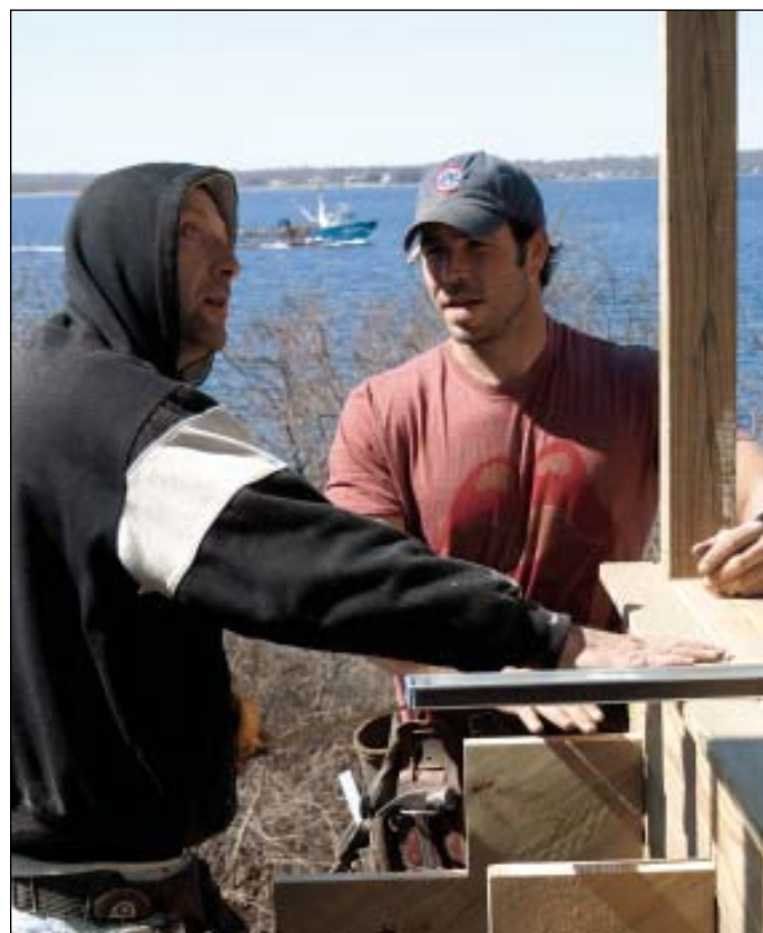
Crew members discuss a framing detail on one of DiGiammo's waterfront condominium projects in Fall River, Mass. On complex residential projects, DiGiammo prefers the efficiency of a crew who knows the more intricate details by heart.
