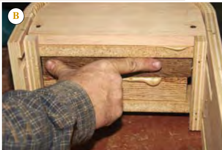
Figure 3. The bullnose riser assembly (A) should be solidly filled to provide maximum holding power for the newel post. The author cuts filler blocks to eliminate all recesses, sliding them into place on a heavy bed of construction adhesive (B).
