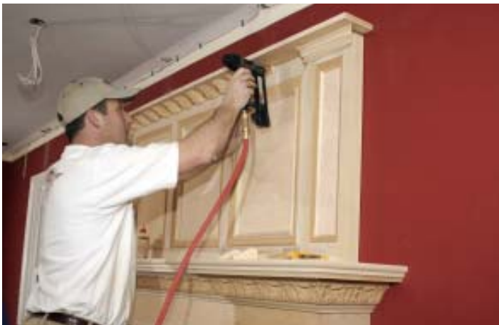
Figure 9. After installing the paneled overmantel (top), the author completes the basic surround by installing cleats and the upper pilasters (center). Then it's time for the finishing details, such as the dentils and moldings that hide the upper shelf joint (above).
