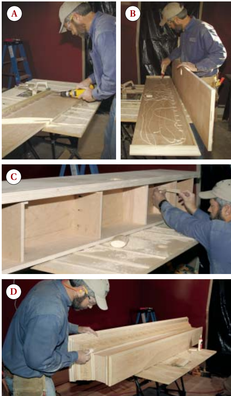
Figure 6. The top of the box — the actual shelf — consists of two layers of \frac{3}{4} -inch plywood. The bed molding that conceals the end joint is securely fastened from behind with pocket screws through the underside of the top layer of plywood (A). Glued into place, the second layer of plywood adds mass to the shelf and conceals the pocket screws (B). The cutouts will accommodate an electrical box. The author fastens the top to the box (C), then finishes the mantelshelf with crown molding (D).
