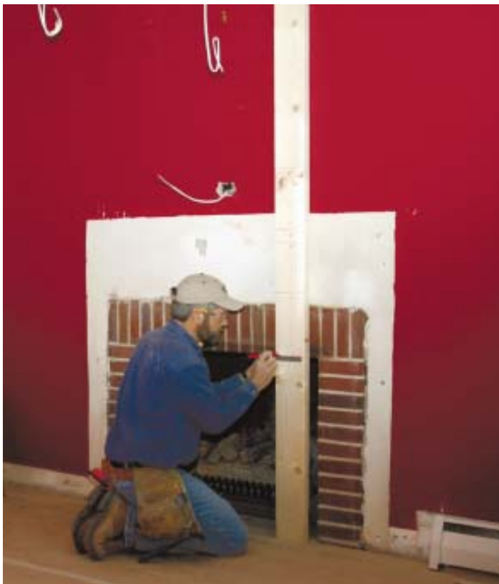
Figure 1. The author starts by marking existing conditions on the story pole, such as the width and height of the firebox opening, the size of the noncombustible material surrounding it, and the proposed height of the mantelshelf (top). Horizontal layouts start in the middle and work outward. Vertical layouts originate from the proposed location of the mantelshelf, go down to the floor, and then work from the shelf up to the ceiling (above).
