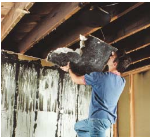
Figure 4. Heat and smoke can travel along joist bays and melt electrical wiring without causing obvious structural damage. Removing drywall is the only way to accurately trace a fire's path and assess the damage.
