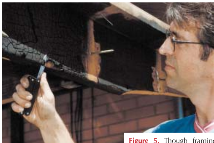
Figure 5. Though framing may be charred on the surface, joists (above) and studs (left) can still be structurally sound. Paring down to solid wood helps the author determine if joists and studs meet code-specified notching guidelines, or if they need replacement.
