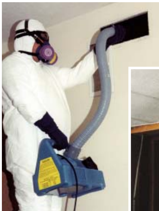
Figure 10. To attack odor-causing particles hidden in wall and ceiling cavities, the author uses a wet fogger to spray a combination of deodorants and sealers through holes punched into the drywall (right). A wet fogger can also be used to deodorize and seal smoky ductwork, though cleaning the ducts properly requires specialized duct brushes and vacuums, a process the author subcontracts (above).
