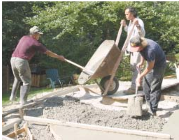
Figure 7. When the concrete can't be poured from the truck, it's transported in wheelbarrows and placed a section at a time.
