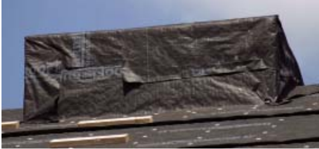
Figure 1. Building the cupola to fit a preframed base made flashing and installation simple. The base was framed with 2x4s capped with a double plate, then sheathed, step-flashed, and papered.
