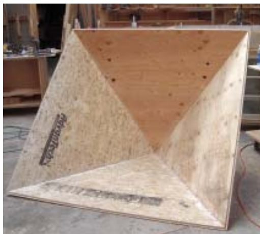
Figure 5. Look, Ma, no rafters! The plywood roof panels are held together with two-part epoxy and a few brads (right). After the epoxy cured, the author glued solid lumber backers along the joints for added strength (far right).
