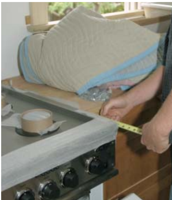
Figure 11. Freestanding stoves should be installed before templating. Otherwise, there could be an uneven gap between the stove and counter. The fabricator is measuring to see if the stove is square to the opening.
