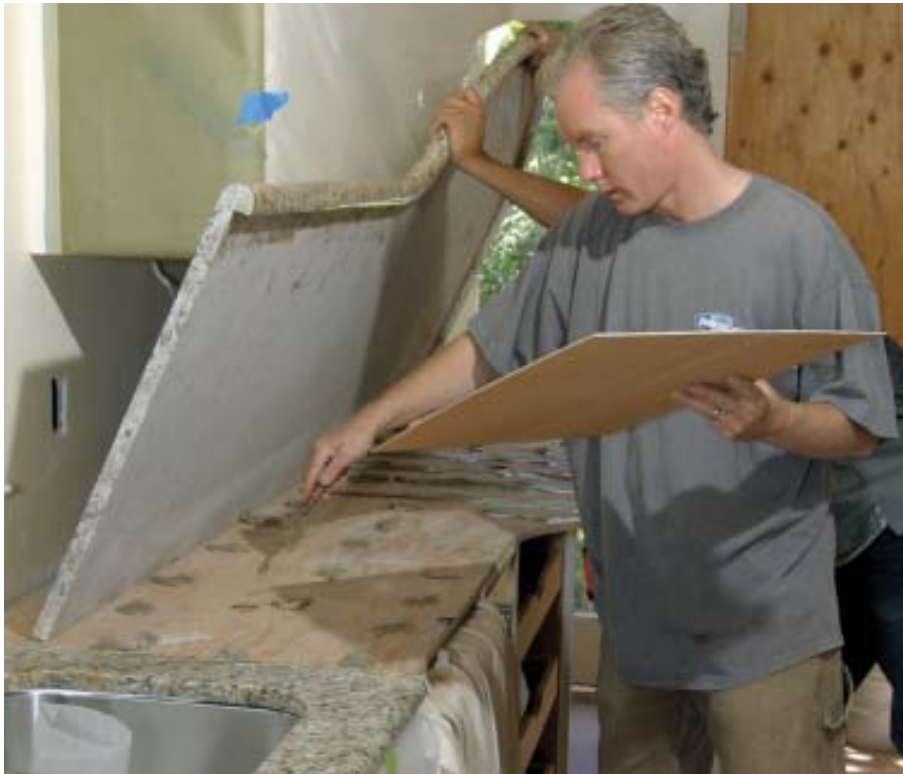
Figure 1. Counters are transported to the site in sections and glued to a plywood subtop with thick dabs of epoxy. This counter is made from 1\frac{3}{16} -inch material. There would be no need for a subtop if it were made from 1\frac{1}{4} -inch structural stone.
