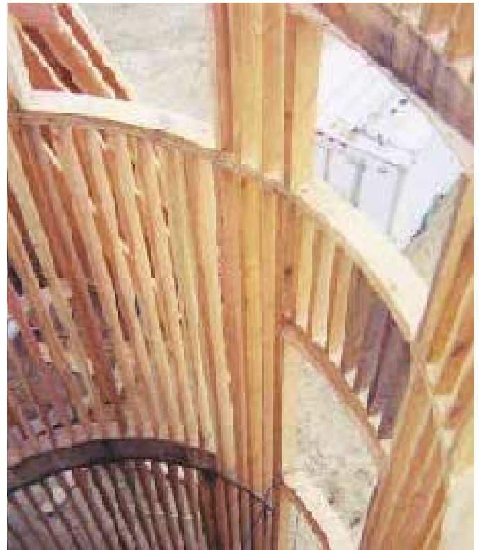
Figure 2. Two layers of \frac{3}{4} -inch plywood, glued and nailed together with overlapping joints, formed the top and bottom plates of the tower's frame (upper right). The sill plate (upper left) was made from pressure-treated plywood. The walls were assembled in place in three sections, with 2x6 studs toe-nailed in place on 6-inch centers, measured along the outside edge (above).
