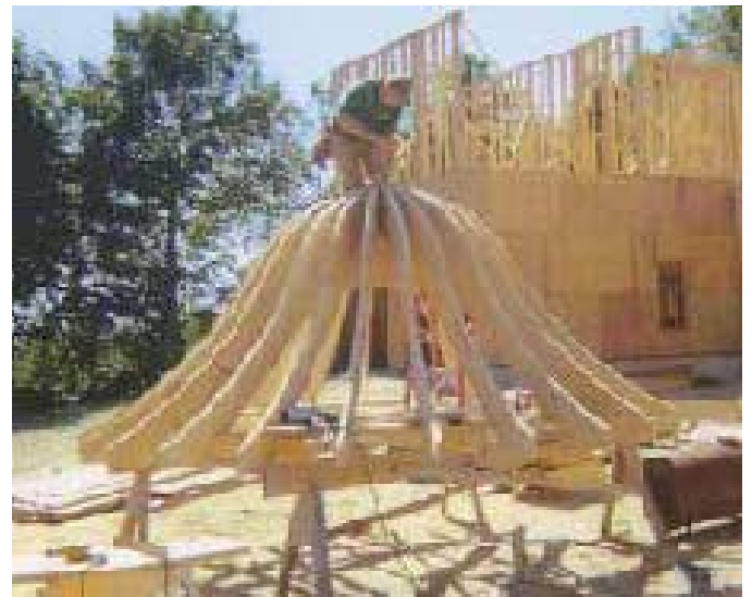
Figure 7. Turret roof framing began with a pair of interlocking rafter pairs on a round plate (top left and right). Intermediate rafters were then filled in (above).
