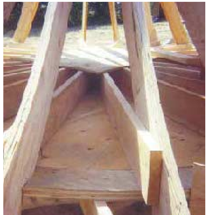
Figure 9. The tower's ceiling joists fanned out from a center triple-2x8 cross member (top left). The birdsmouths were cut loose (top right) to allow the roof to slip into place over the sheathing lip described in Figure 5. The eventual ceiling surface was backed with 1/2-inch plywood (above) to stiffen the roof assembly for lifting, as well as to provide nailing for the radius crown molding.
