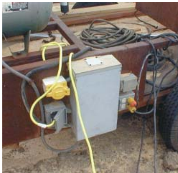
Figure 4. An electrical distribution box supplies power to the tools on and around the trailer. The duplex receptacles are wired to a GFI breaker and the box itself is connected to a power pole.
