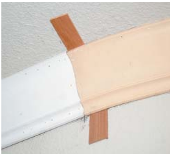
Figure 4. MDF is often thicker than flexible molding, so shims placed behind the flexible molding smooth the transition.
