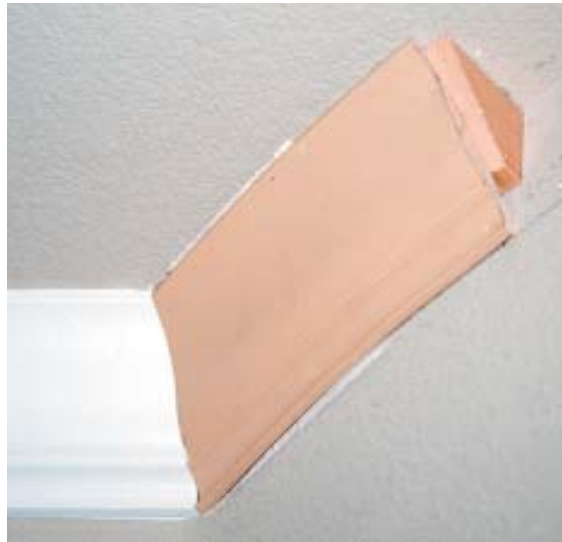
Figure 3. Triangular blocks keep the crown from bowing in, provide nailing at joints, and make transitions to regular crown molding easier.
