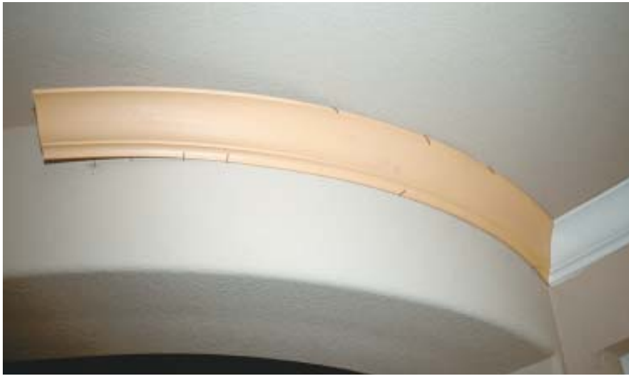
Figure 2. Finish nails help hold the crown in place and free a hand for operating a nail gun. Because the author uses MDF moldings, inside corners are mitered not coped.
