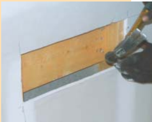
Adding missing blocking for a stair rail rosette from the back of the wall produces an invisible patch.
