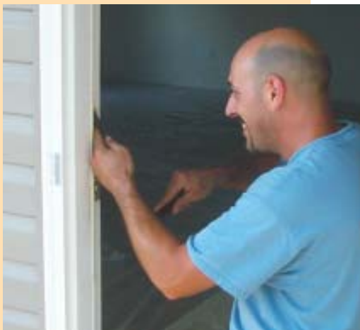
Lockout crews install door and other hardware and fine-tune the finished job.
