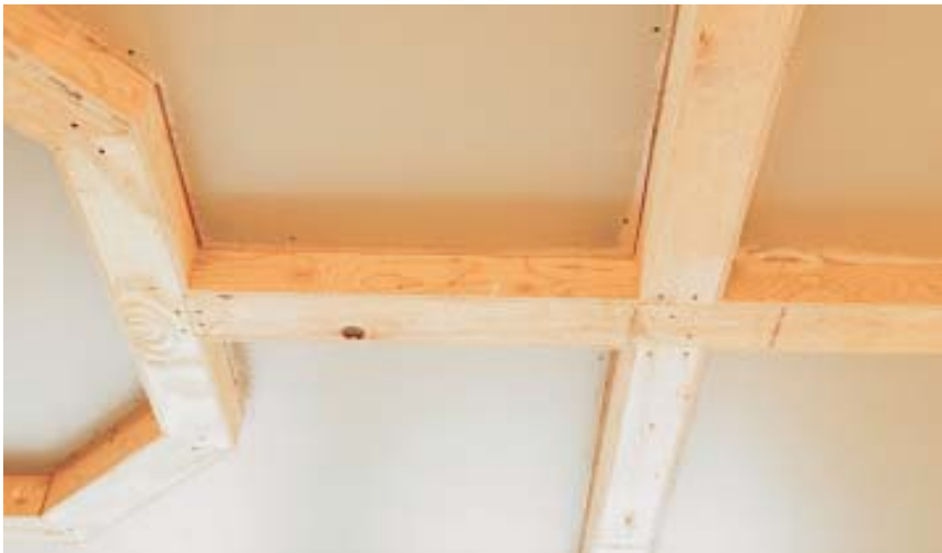
Figure 2. Half-inch or \frac{3}{4} -inch plywood strips screwed into the nailers form the sides of the beams. The bottoms of the plywood boxes are \frac{3}{4} -inch for easier fastening. Because it is so dimensionally stable, the plywood substrate helps to prevent gaps in the finish lumber.
