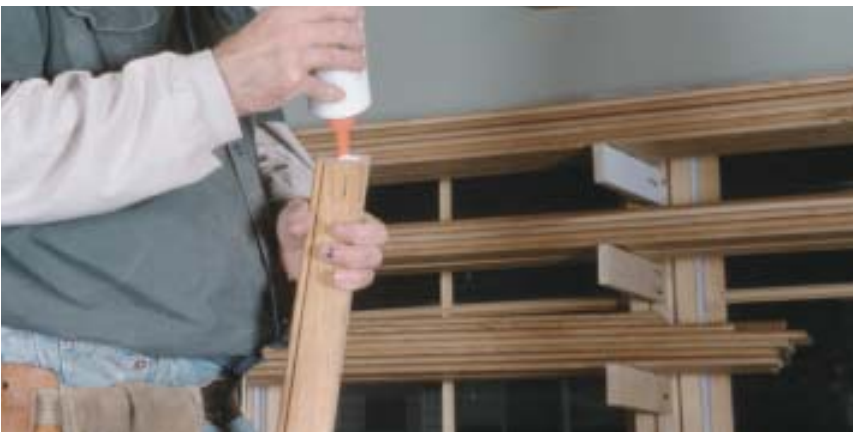
Figure 5. Storing the beam stock on high cleats keeps it in easy reach of a carpenter working from stilts.
