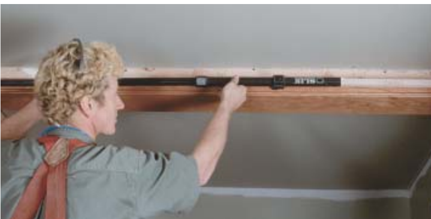
Figure 6. A telescoping leg from a camera tripod serves as an accurate inside-dimension measuring tool. The leg is locked into place, then handed down to the carpenter making the cuts.
