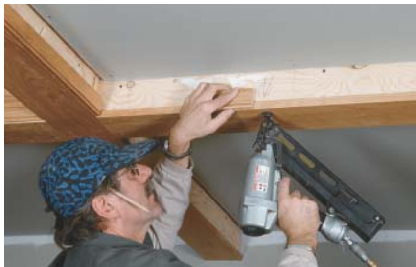
Figure 3. A Bosch miter finder helps achieve a perfect joint at beam intersections (top), while biscuits help prevent the joints from moving over time (center). The carpenter uses a scrap of the side material to help center the bottom piece (bottom).
