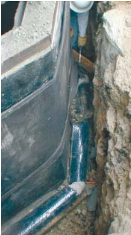
Figure 10. Formed shotcrete walls are waterproofed with a layer of Paraseal membrane — visible near the top of the wall — followed by dimpled drain mat. The upper edge of the drain mat will be secured with a termination bar provided by the manufacturer. The worker visible at top is standing in an excavated void reinforced with stitch piers.
