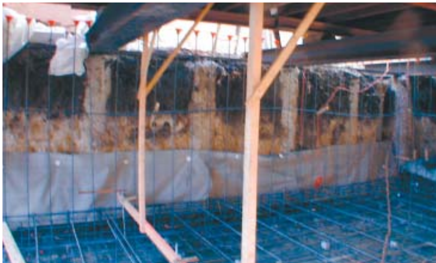
Figure 8. A two-layer rebar grid reinforces the structural slab against seismic loads and eliminates the need for pad footings beneath point loads. After the slab has been poured, drain mat and waterproofing membrane will be applied to the face of the excavation — which has been stabilized with stitch piers — and shotcrete will be gunned against the bank. The above-grade portion of the wall will be backed by a single-sided form. To avoid puncturing the slab membrane with grade stakes, the screeds that will be used to level the slab are supported with temporary lumber braces nailed to the overhead joists.
