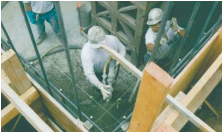
Figure 9. Gunning shotcrete against a single-sided form, rather than directly against the excavation, provides space for stone backfill and affords more control over the waterproofing on difficult sites.
