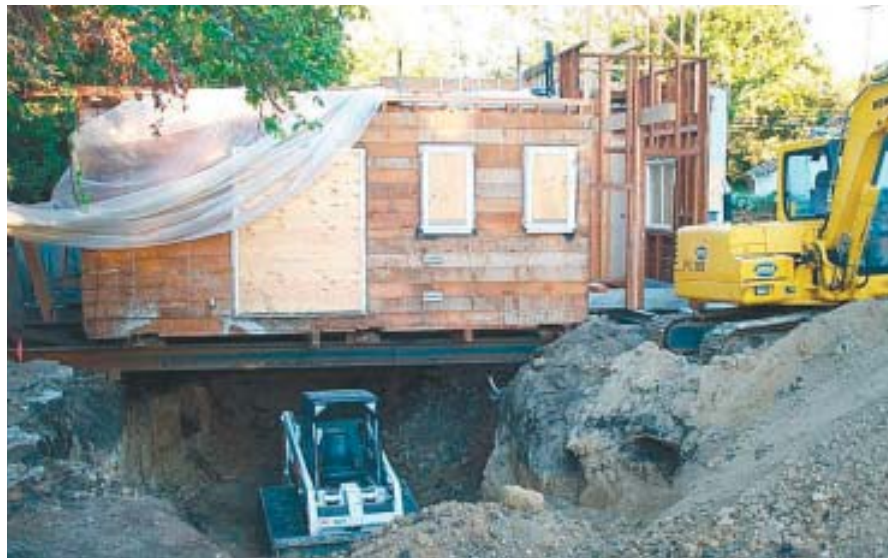
Figure 4. Tracked skid-steer loaders are preferred for working beneath the house because they're highly maneuverable and provide excellent traction. The skid-steer pushes the excavated soil to an opening, where it's scooped up by an excavator and loaded into a waiting dump truck.
