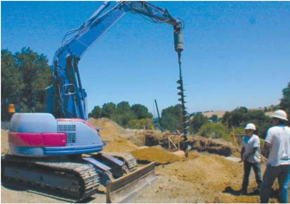
Figure 2. An excavator-mounted “dangle drill” is used to bore holes for stitch piers. Bit extensions can be added as needed to bore to depths of 25 feet or more. The drill rig can also be used to insert rebar assemblies that are too heavy to move by hand.
