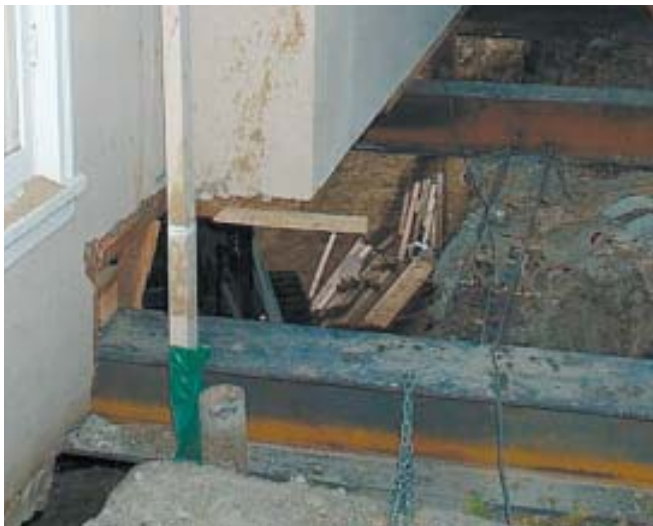
Figure 3. The steel beams that temporarily support the structure are inserted into holes that have been jackhammered through the stem walls. Once the beams have been raised into position with jacks and shimmed into place, the jacks are removed and the original foundation is demolished.
