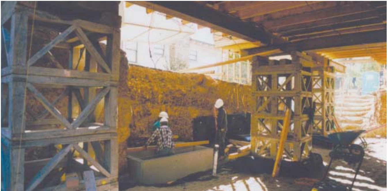
Figure 5. Where full-length shoring beams are impractical, shorter beams are supported by cribwork as needed. No stitch piers were required to support the solid soil forming the face of the excavation shown here. The concrete vault will eventually house a sump pump.
