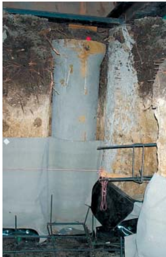
Figure 7. A reinforced concrete pipe set into a groove cut into the excavation face provides a drainage sump that lies outside the living space. The turned-up edge of the slab waterproofing membrane covers the lower section of the pipe, which will later be covered by a reinforced shotcrete wall.
