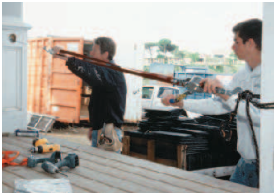
Figure 7. The PVC radius railings rely on a tensioned steel cable for strength (top). A come-along provided the necessary pull (bottom). The 3-inch hole where the cable is cinched will be covered by a removable section of straight railing, should the cable ever need retensioning.
