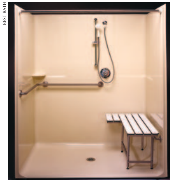
Figure 1. An accessible replacement shower unit may be too large to get through the front door. Many units are available in multi-panel kits for that reason.
