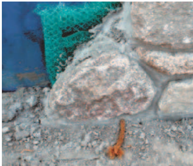
Figure 2. To ensure that any water that penetrates the masonry veneer will drain out again, a narrow void behind the face wythe is protected from mortar droppings by an open polyethylene mesh. The supporting wall has been waterproofed with a sprayed-on membrane. A natural fiber rope wick, inserted at the base of the veneer, prevents mortar from clogging the weep hole.
