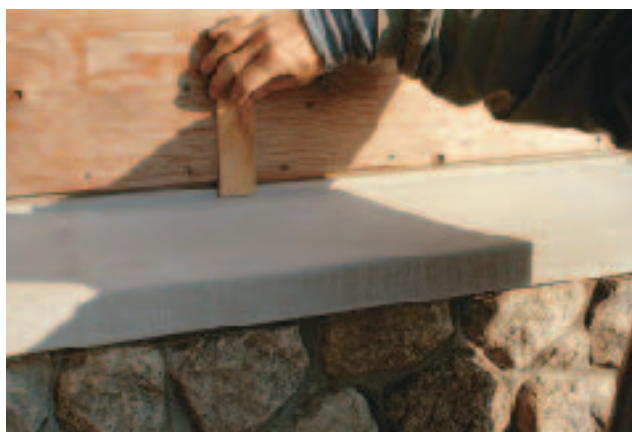
Figure 6. It's important to protect the top of the veneer from water penetration. Here, a sloped limestone cap delineates the transition from stone to wood siding.
