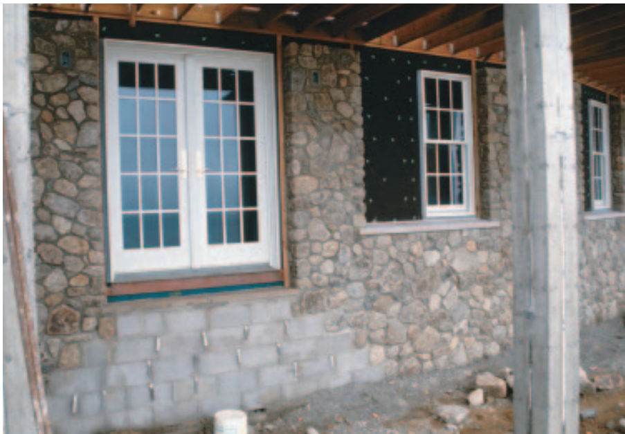
Figure 1. Material and time are saved by using concrete masonry units in areas that will be backfilled or otherwise concealed — in this case, by a fieldstone step.
