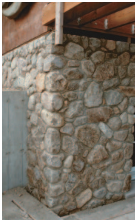
Figure 4. The structural integrity and visual continuity of an outside corner depend on a careful, sequential left and right distribution of stones. This requires both sides of the corner to be worked simultaneously.
