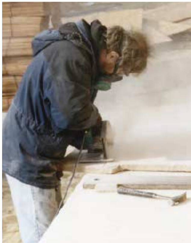
Figure 4. Working from the back of the slabs, the crews used a circular saw equipped with a diamond blade to score the stone most of the way through.
