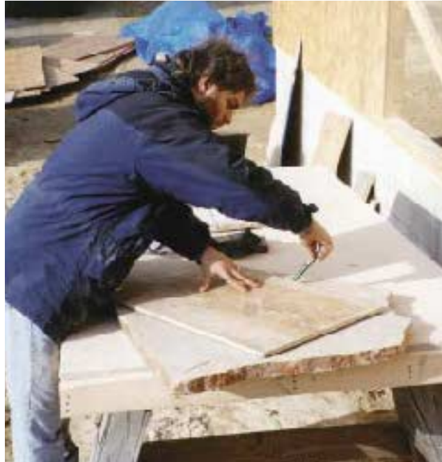
Figure 3. OSB templates assisted in getting the best yield from the stone slabs.
