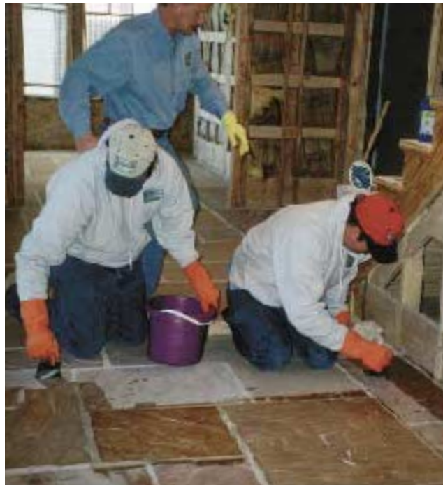
Figure 7. After cleaning the stone with a proprietary cleaner, workers applied two coats of solvent-based sealer and one top coat to finish the job.
