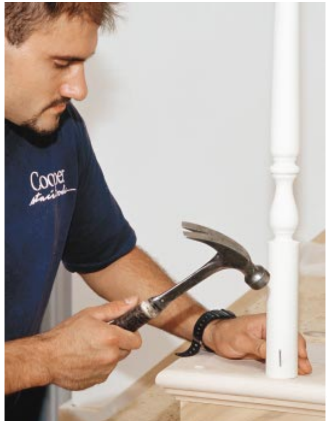
Figure 12. The author fastens the top of the baluster with a 4d finish nail and the bottom with a 6d finish nail.
