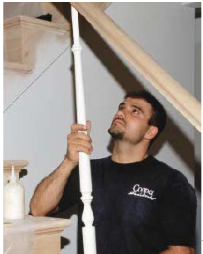
Figure 10. The author slides a baluster into the predrilled hole in the railing, then lowers the pin into the hole in the tread. He sights the rail: It should have a very slight crown.
