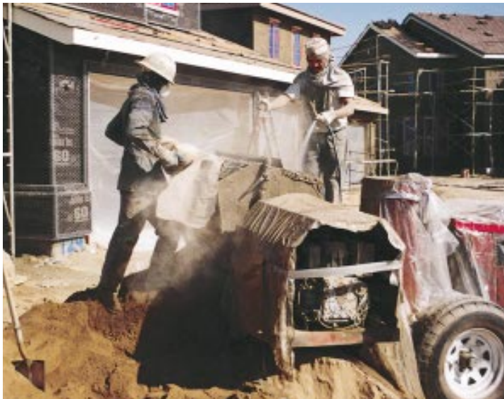
Figure 4. Clean sand, dry cement, and the correct amount of water are key to a good stucco mix.
