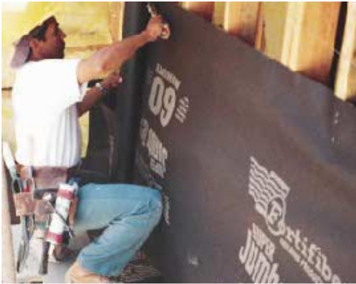
Figure 1. A properly installed weather-resistive barrier is essential to protect the structure from moisture intrusion. Here, 60-minute Type D kraft paper is being installed.
